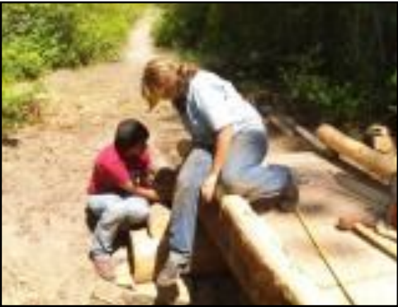
Lynn Kennedy and Jessica Puente put the finishing touches on one of the Whistler Canyon bridges
